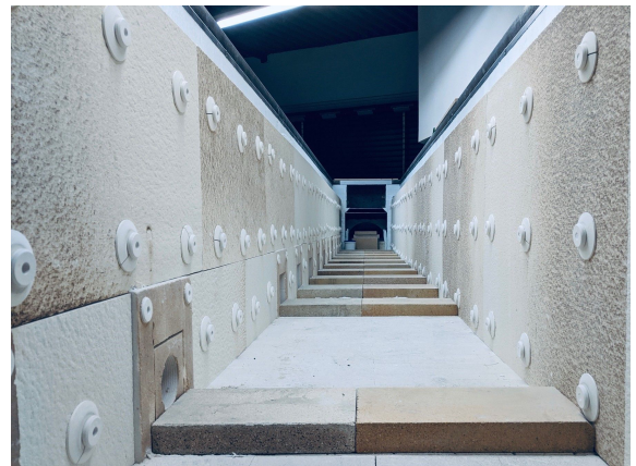
Heat treatment furnace insulation
