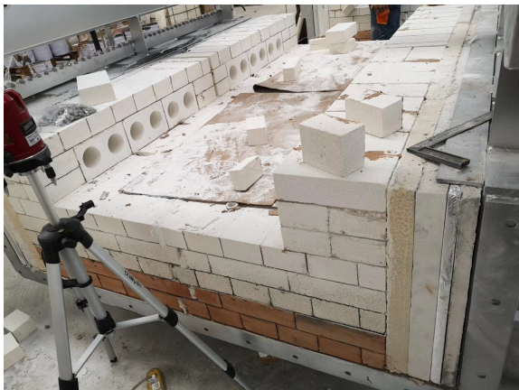
Roller Kiln Backing Insulation
